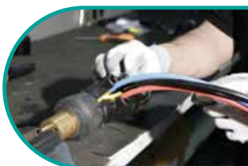
Assistance Technique/ Retrofit
